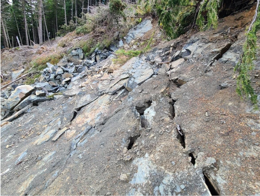
A: Looking east at a dilated rock block in the central portion of the slide near elevation 730 feet.
