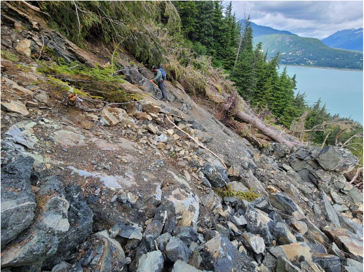
Looking west at a dilated rock block in the central portion of the slide near elevation 730 feet.
