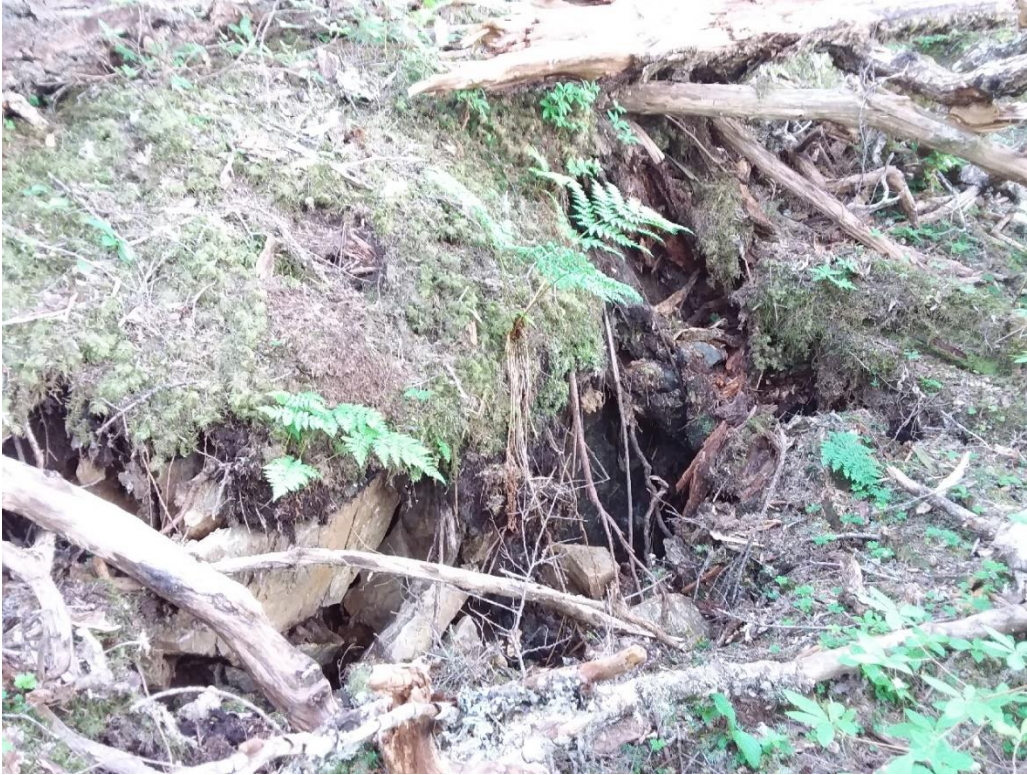
A: Cavities developed along the eastern tension crack.
