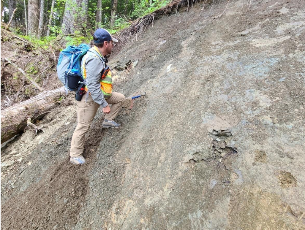
A: Looking southeast at the eastern extent of the headscarp (at the highest elevation).
