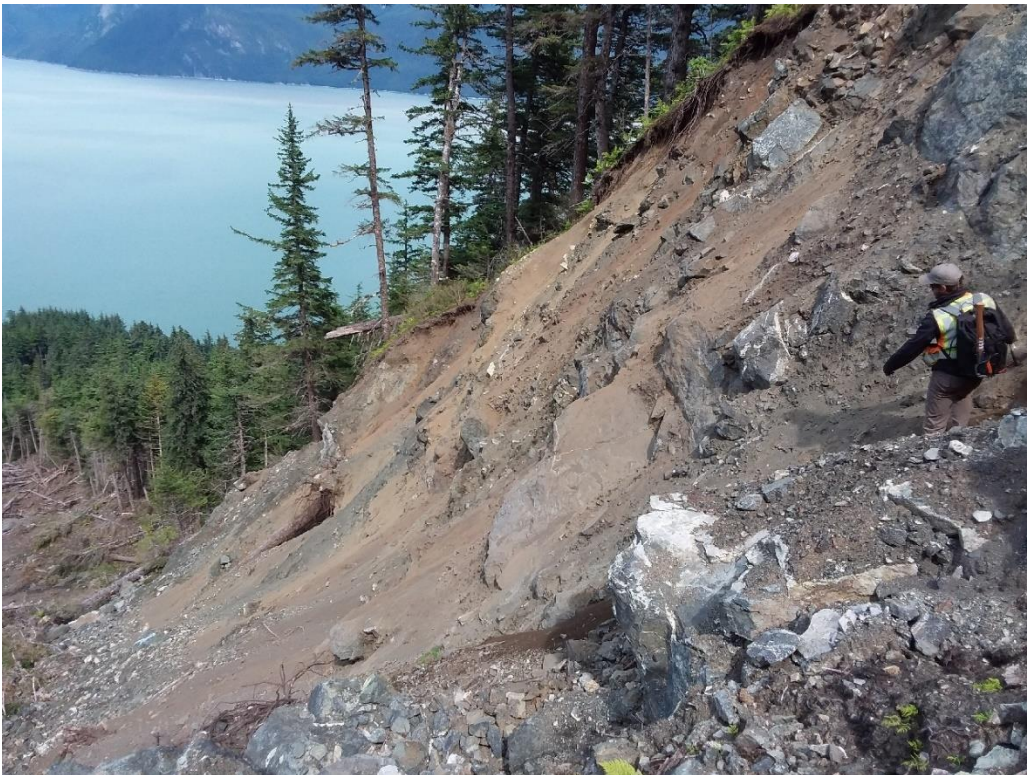
B: Looking northeast at the eastern lateral soil scarp below elevation 800 feet.
