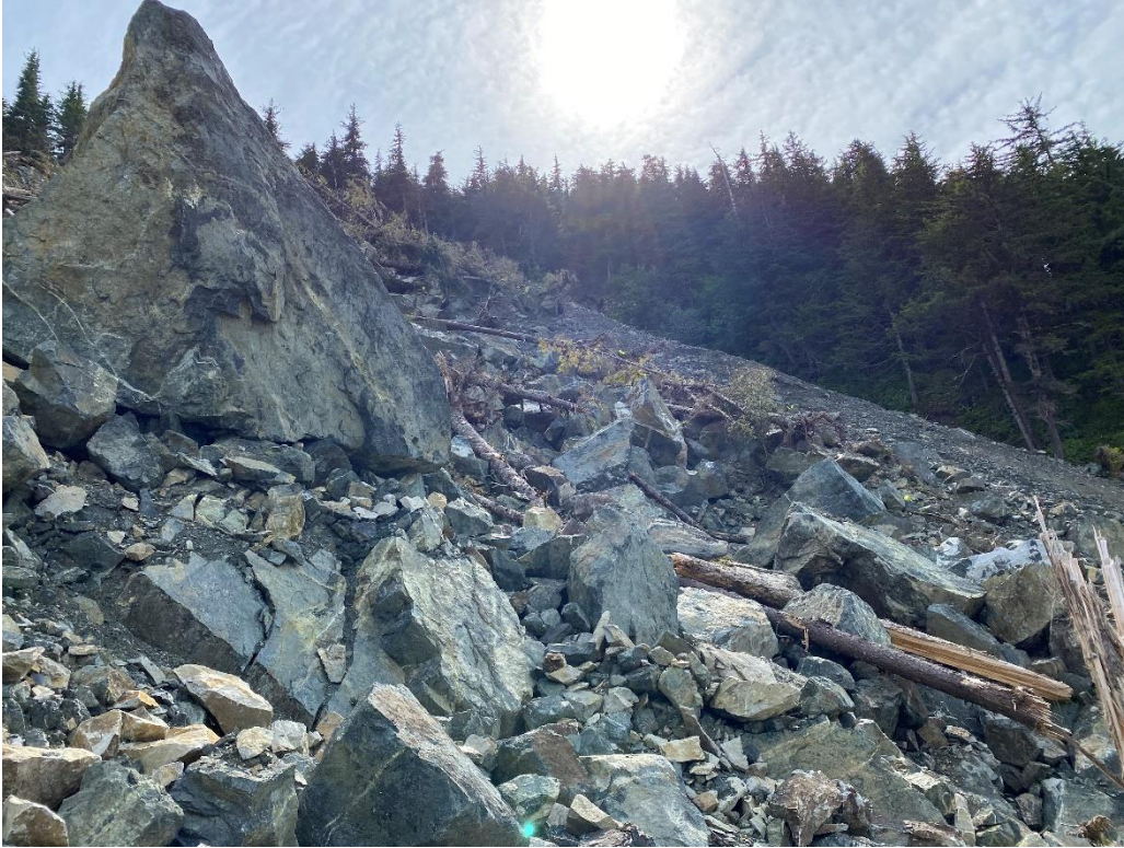
A: Looking southwest at the boulder field in the main body of the slide.
