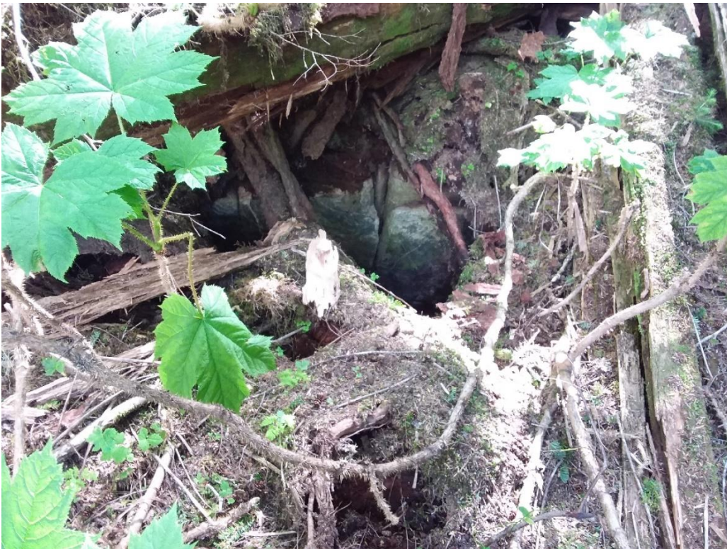
B: Looking southwest at an eastern tension crack cavity, approximately 150 feet from the headscarp.
