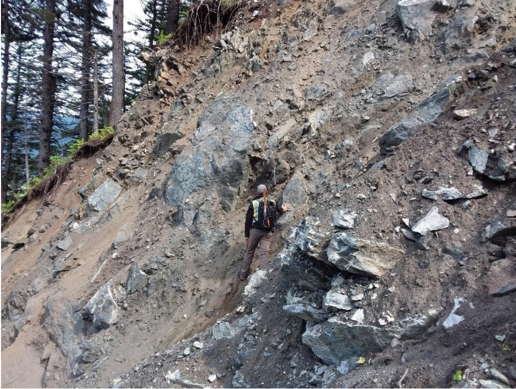
A: Looking east at the eastern lateral soil scarp below elevation 800 feet.
