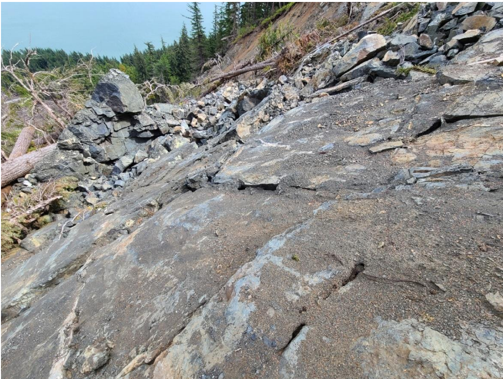
B: Looking northeast at a dilated rock block in the central portion of the slide near elevation 730 feet.
