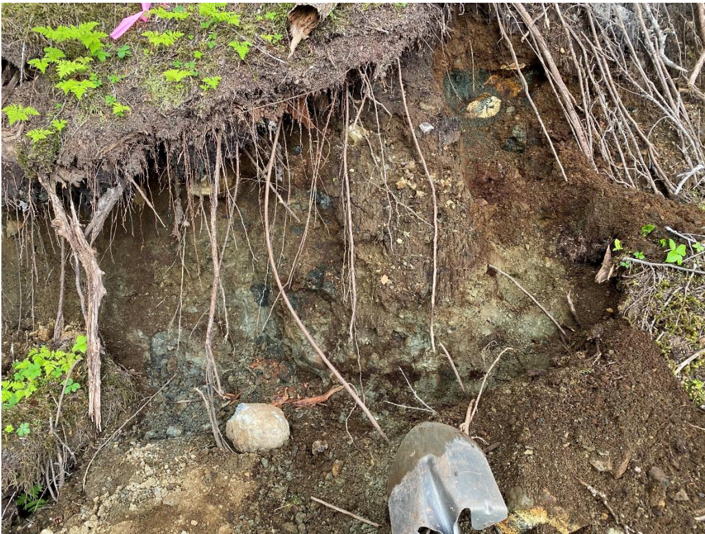
B: Eastern tension crack with roots pulled in direction of movement.
