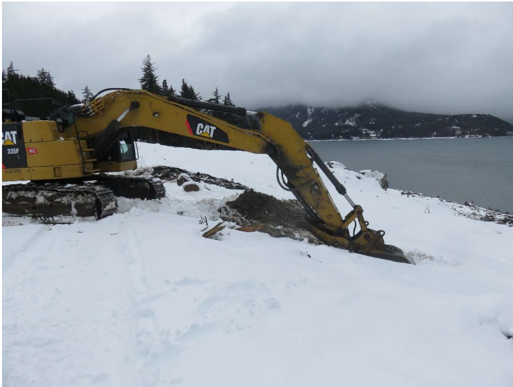
View of excavator excavating a test pit (TP-2) on the east end of the temporary access road (taken 2/27/2021).
