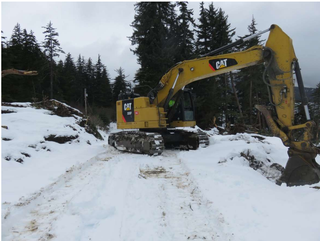
View of excavator excavating a test pit (TP-4) on the west end of the temporary access road (taken 2/27/2021).
