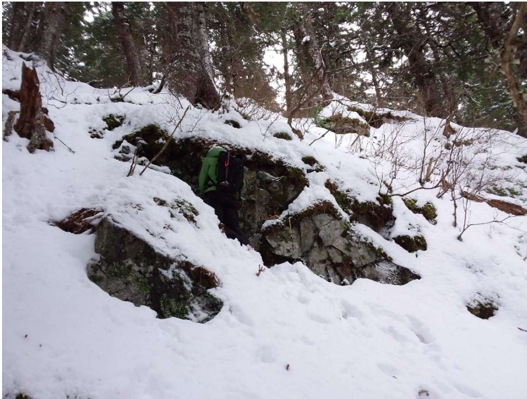
View looking southwest at rock outcrop above the prominent rock knob just east of the slide. The rock appears to be in place (taken 2/26/2021).
