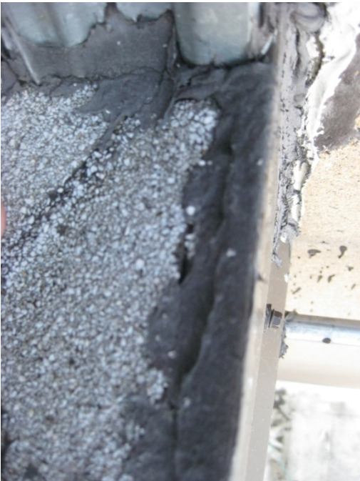
Leak point at adjacent structure.
