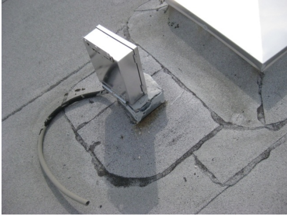
Failed pitch pocket.
