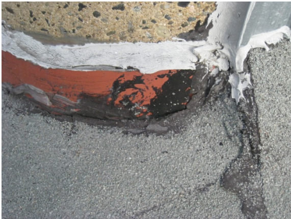
Leak point between pool roof and concrete wall.
