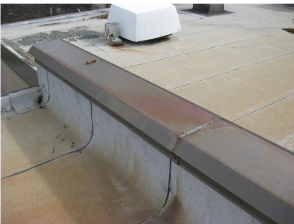
Rust stain at parapet.
