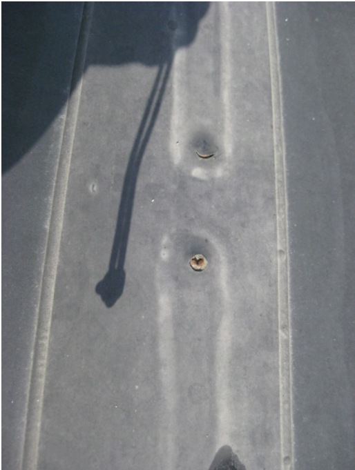
Membrane damage at protruding fasteners.
