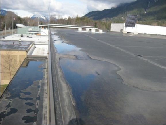
Area where soft roof substrate was encountered.
