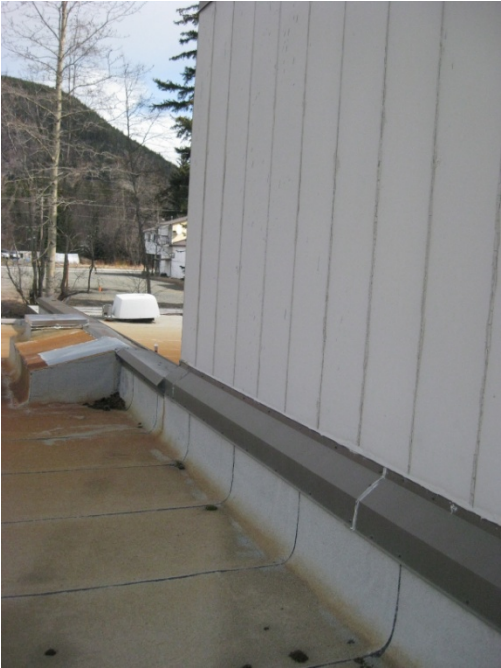
Potential leak point at wall seams.
