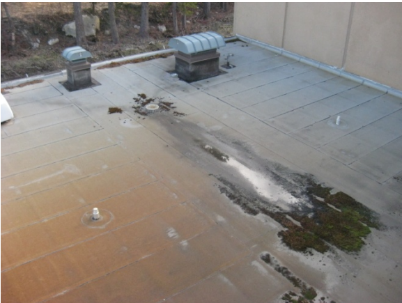
Overall view of Area 4. Roof with moss buildup at roof drain.
