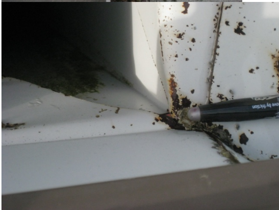
Leak point in gutter.
