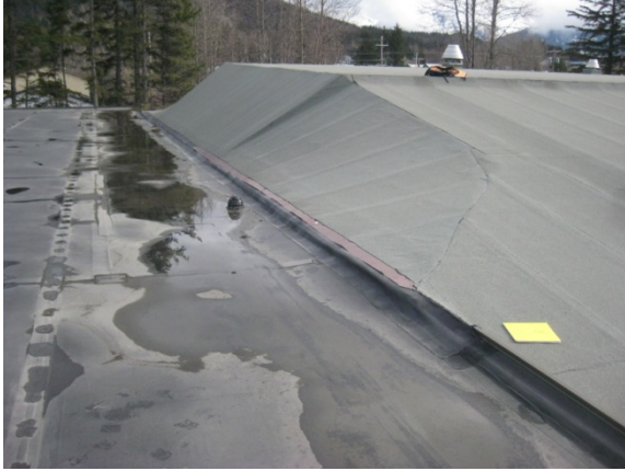
Potential leak point between gym roof and pool roof.
