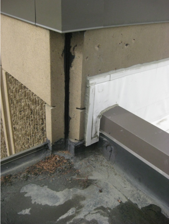
Potential leak point at intersection with music room.
