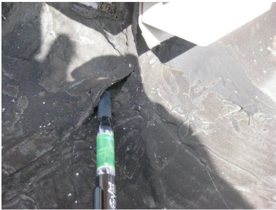
Seam failure at exhaust cap.
