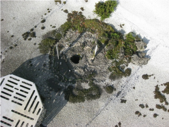
Moss buildup at roof drain.
