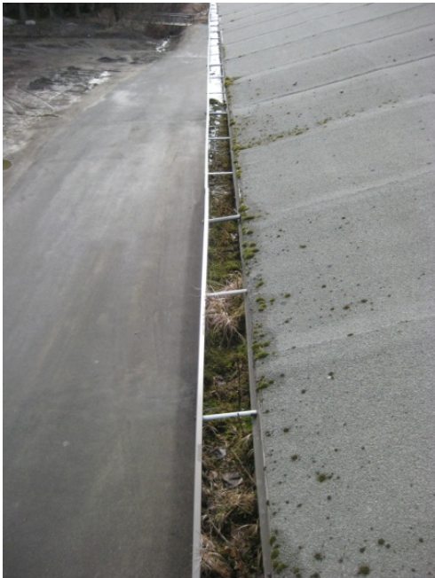
Moss filled gutters.
