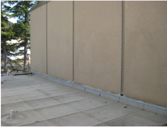
Potential leak point at concrete wall.
