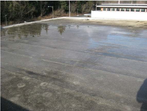
Overall view of Area 4 with ponding evident.
