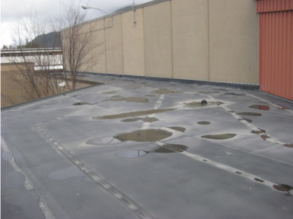
Overall view, low roof at entry hall – note ponding
