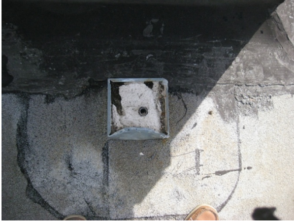
Failed pitch pocket.
