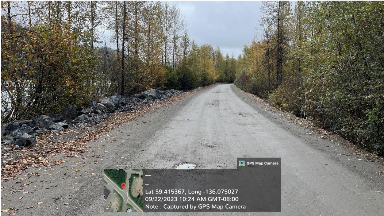
Figure H.1 – Riprap on left was placed in 2022 as described in FH22-I-0090. This is the same location as 2023 Third-Party Work Site 1. Third-party work placed 3’ of road fill up against backside of riprap berm placed in 2022.
