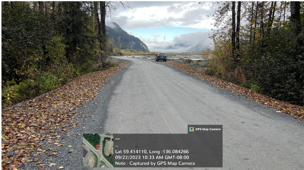
Figure A.5 - Porcupine Trail Road Phase I stop of work, photo facing end of road. Also shown is start of third-party Site 2 work. This location is near the start of yet to be designed Phase II work.
