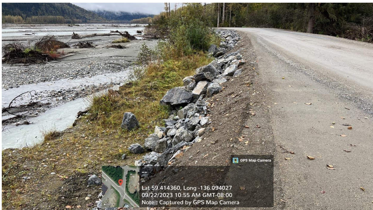
Figure C.9 – Riprap placed at third-party work site 3 on Klehini River side of roadway fill slope above ordinary high water. Note the presence of existing uplands vegetation between toe of fill and river, as well as the existing undisturbed roadway grade at toe of fill in foreground.
