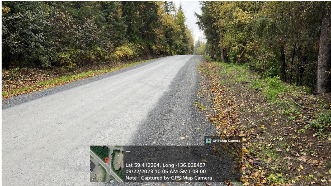
Figure A.1 – Porcupine Trail Road Phase I start of work, photo facing end of road. Begin Phase I project.
