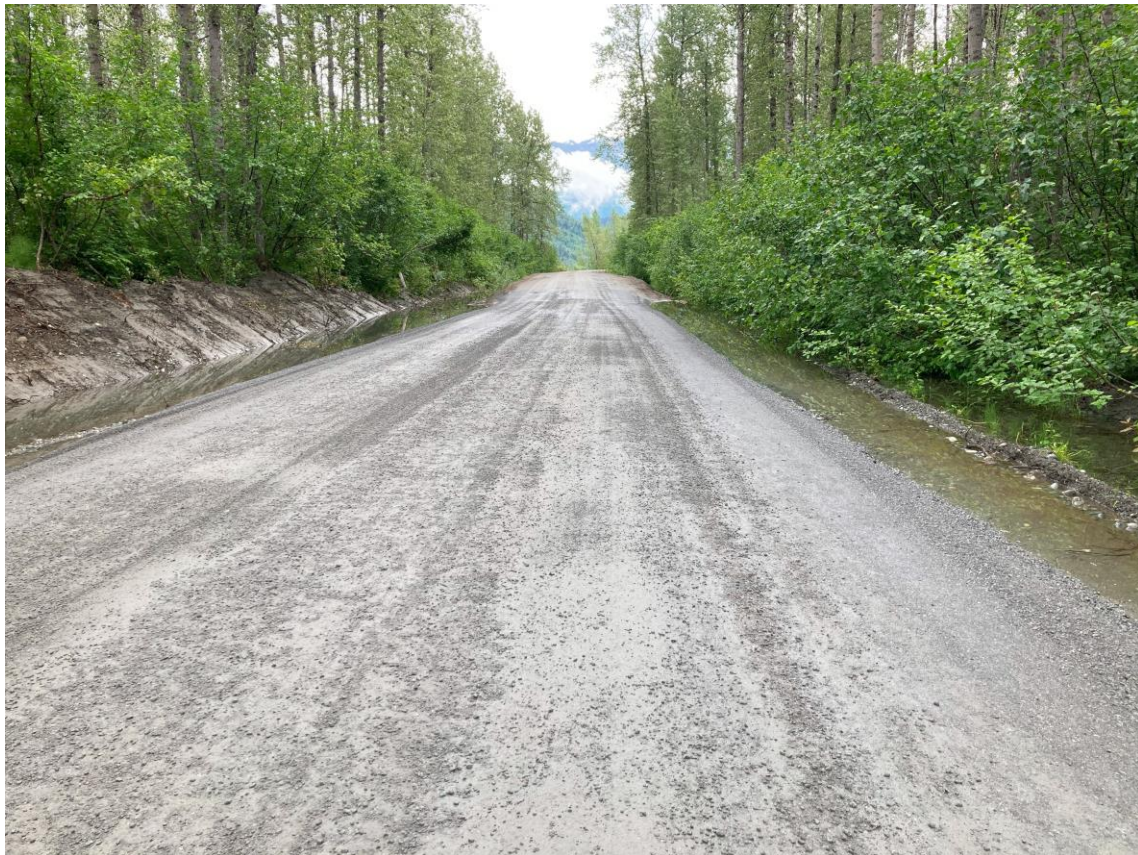
Area that water exceeded ditches
