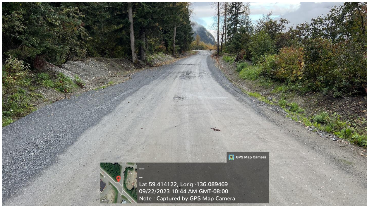
Figure A.6 - Third-party stop of work for Site 2, photo facing end of road. Also shown is start of a short section of Porcupine Trail Road Phase I work, approximately 300' segment between end of third-party Site 2 work (foreground) and beginning of third-party Site 3 work (distant background).
