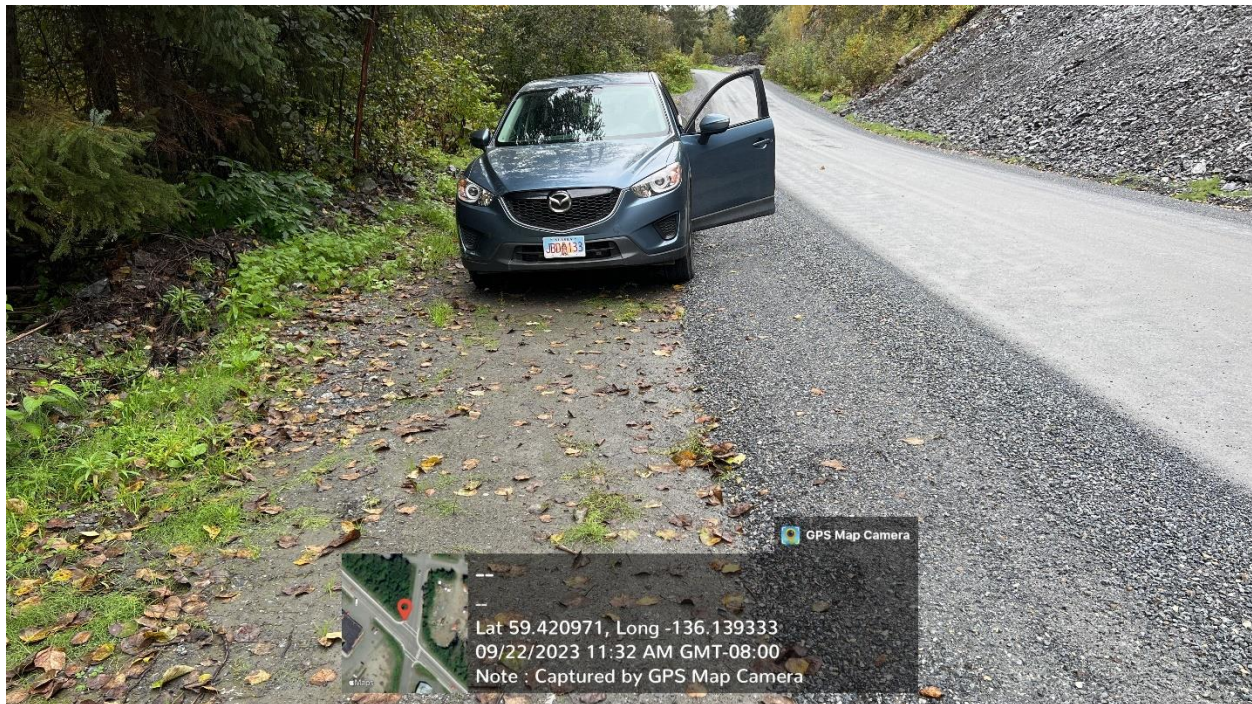
Figure F.2 – Typical existing pullout on Porcupine Trail Road within the Phase I work limits where gravel surfacing was placed per Plan and did not extend to the limits of the existing roadway.
