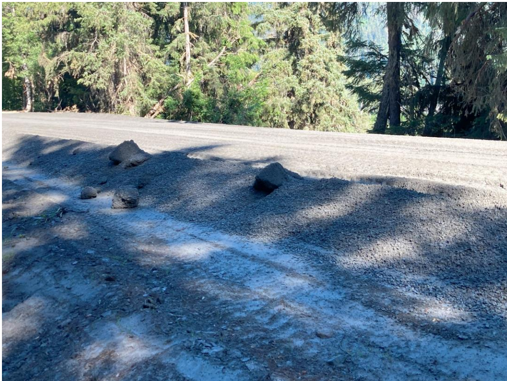
Worst of the clumps of Calcium Chloride
