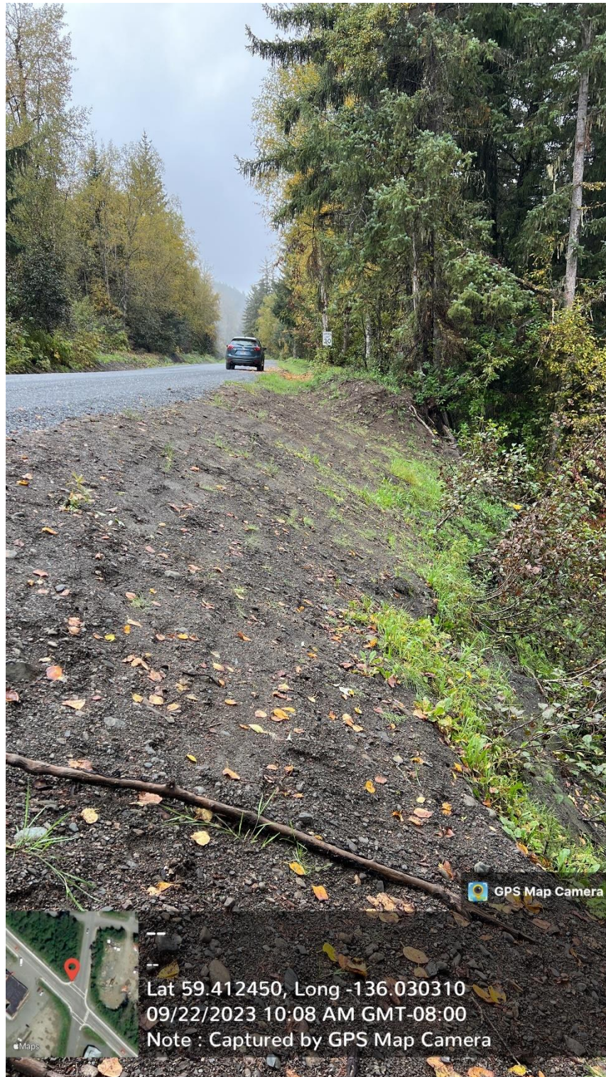
Figure F.1 – Performed as part of Phase I work, ditch and roadway reconditioning spoils were placed on the downslope side of the existing Porcupine Trail Road corridor to facilitate positive drainage from roadway surface and ditch in background of photo. Roadway reconditioning removed an existing berm along the edge of the road which blocked surface drainage and spread it downslope as shown.
