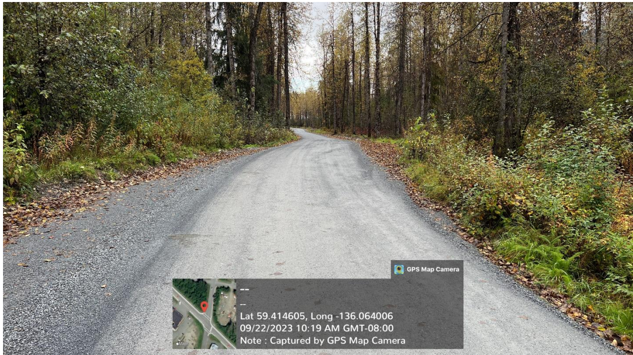
Figure E.1 – Phase I gravel surfacing work at Herman Creek, culvert crossing at photo center, photo facing end of road.
