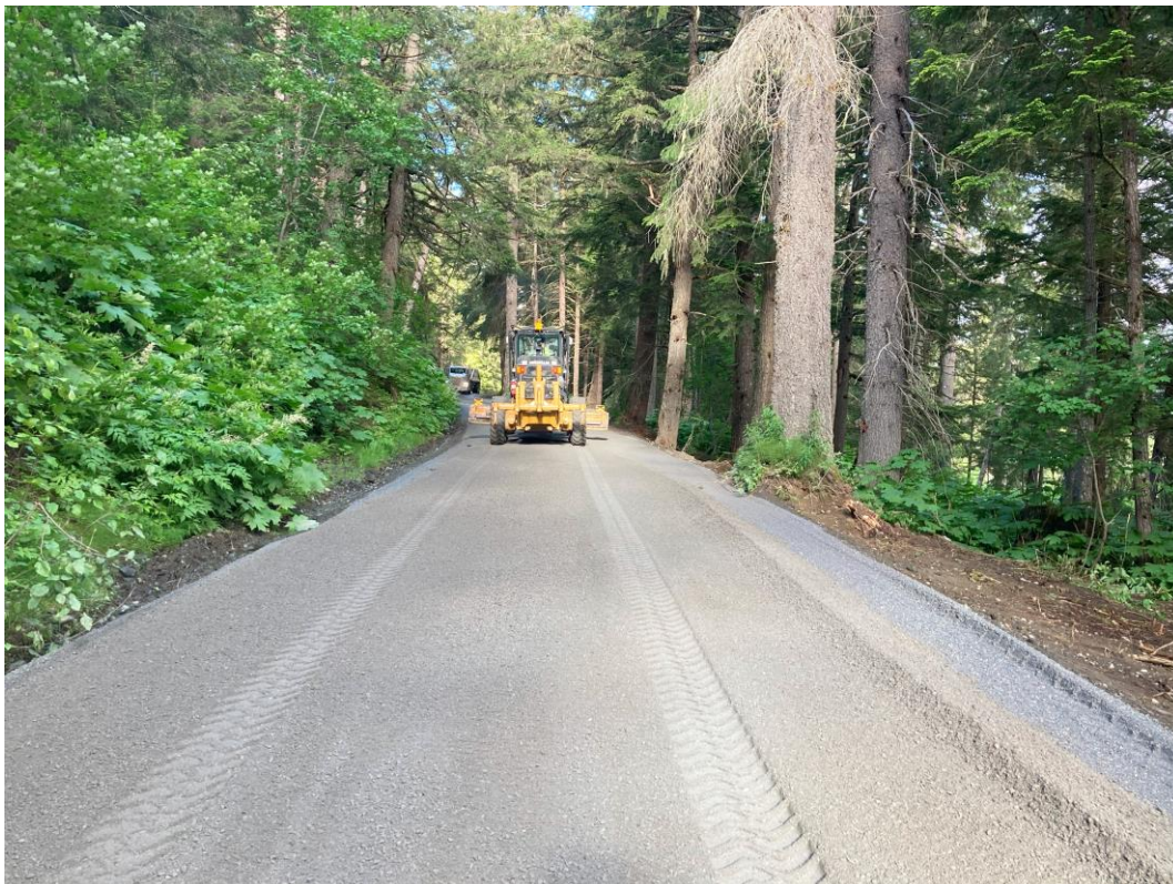
Cat 12 Grader set back to beginning of last section to start the 2 nd lift with Calcium Chloride
