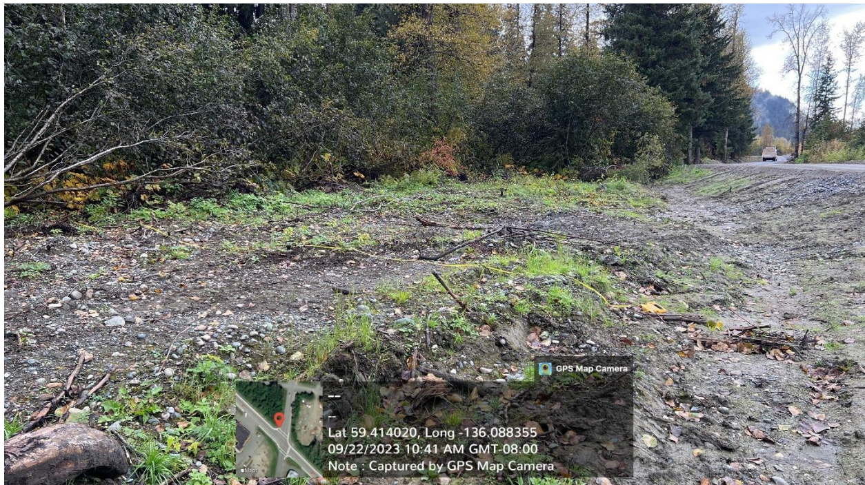
Figure H.5 – Area adjacent to Porcupine Trail Road and Third-Party Work Site 2 where a significant amount of gravel and debris were deposited during flood events. Area appears to be disturbed because it was used as a source of material to construct gravel/debris berms described herein and FH22-I-0090.
