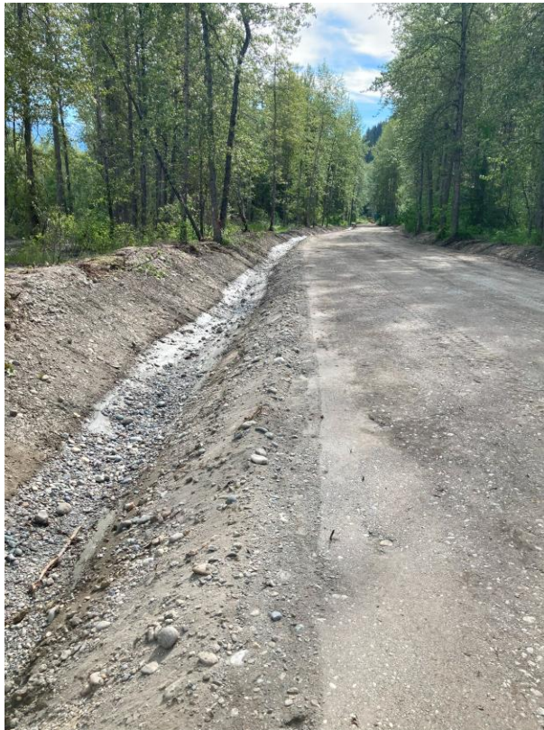
Water line from yesterday
