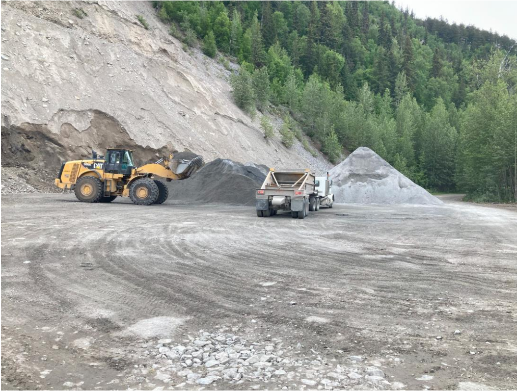
Calcium Chloride material stockpile is running low.
