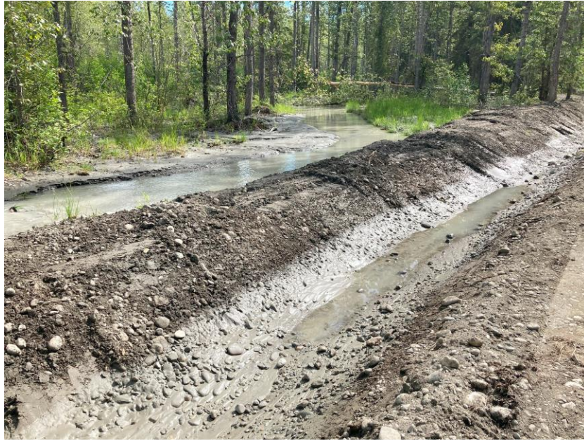
Water flow above the right ditch
