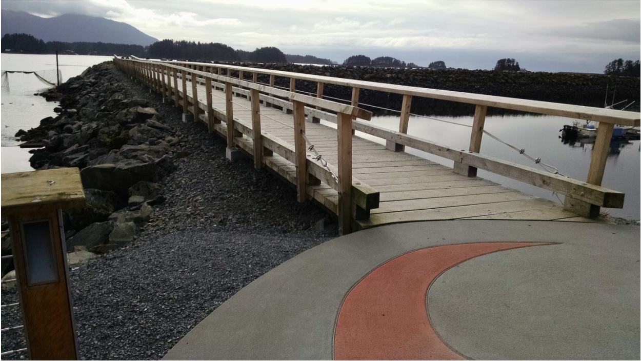
A simple boardwalk built on top of the rubble mound breakwater leads to a lookout of Sitka Sound.
