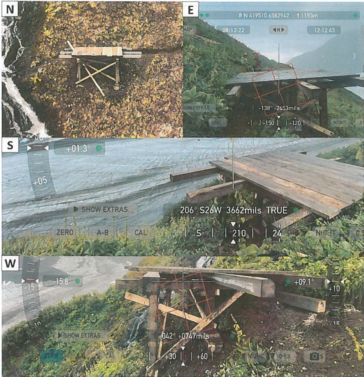
Photo 23: Cantankerous Pump (CAP SE) Pad post-build. Cantankerous Pump was used to source water for 2022 Paradise City drill pad holes. Pad retains full decking and remains unreclaimed for potential future use.
