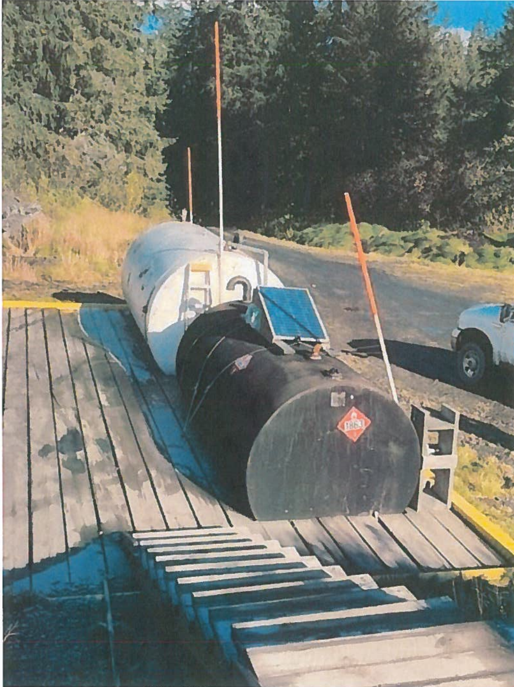
Photo 1. Fuel Station at the Glacier Creek Laydown. Tanks were emptied and winterized in October of 2022 (Photo: Oct 2021).
