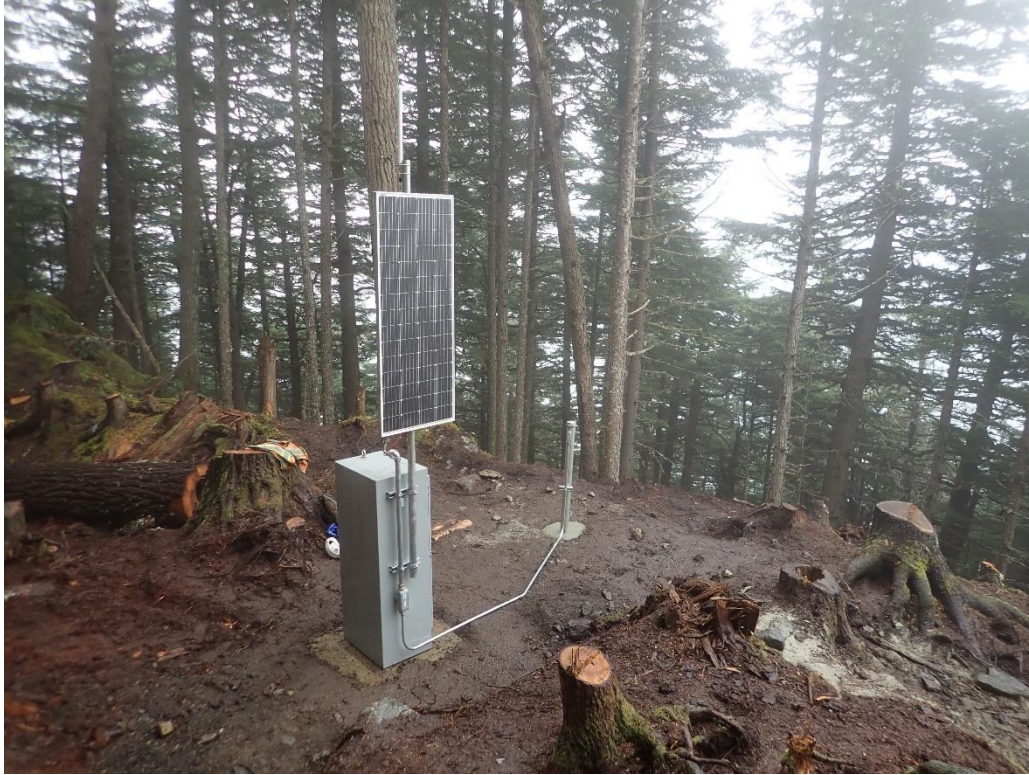
A: Typical instrumentation installation: free-standing enclosure with solar panel (LT-9)
