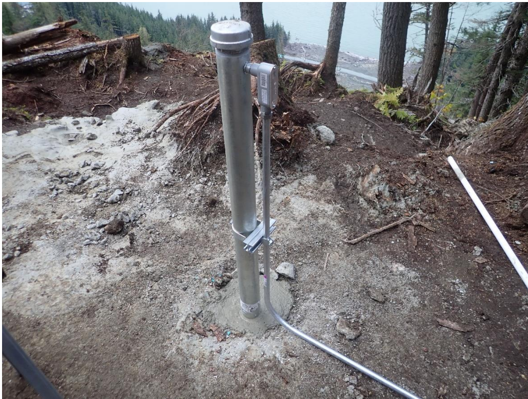
B: Typical monument completion housing SAAV and VWP cables
