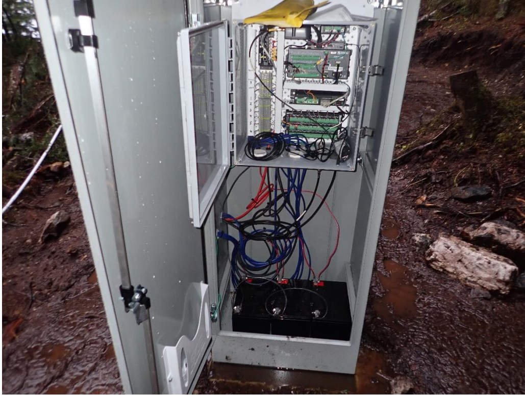
A: Inside free-standing enclosure of base station installation at LT-6
