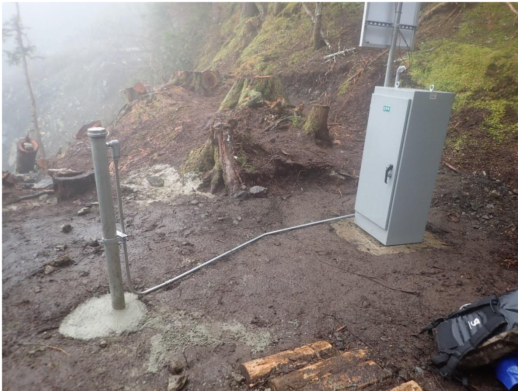
B: Typical instrumentation installation (LT-9)
