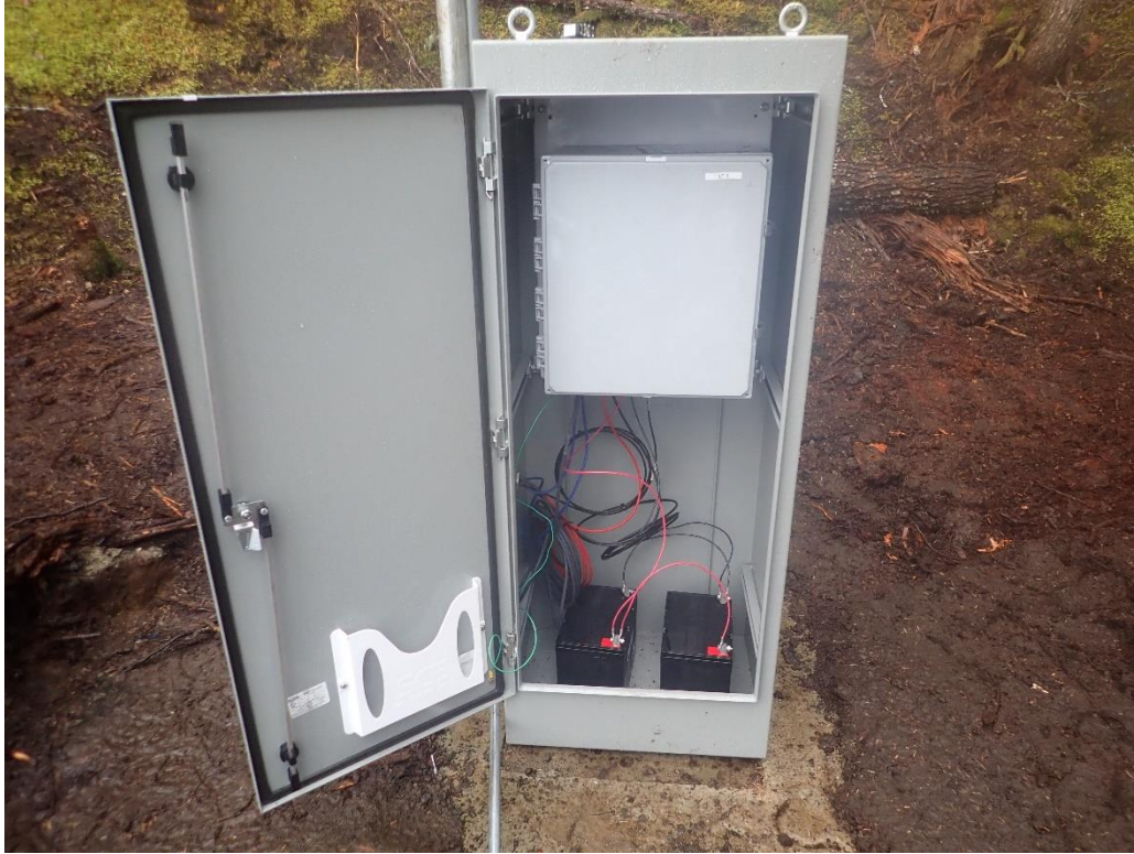
A: Typical free-standing enclosure installation with batteries and secondary enclosure
