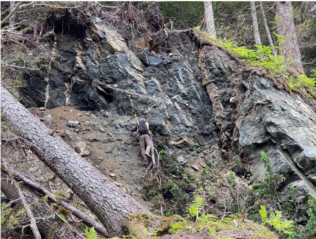
B: Rock 2 located at elevation 820-840 feet on the west headscarp of the 2020 landslide.
