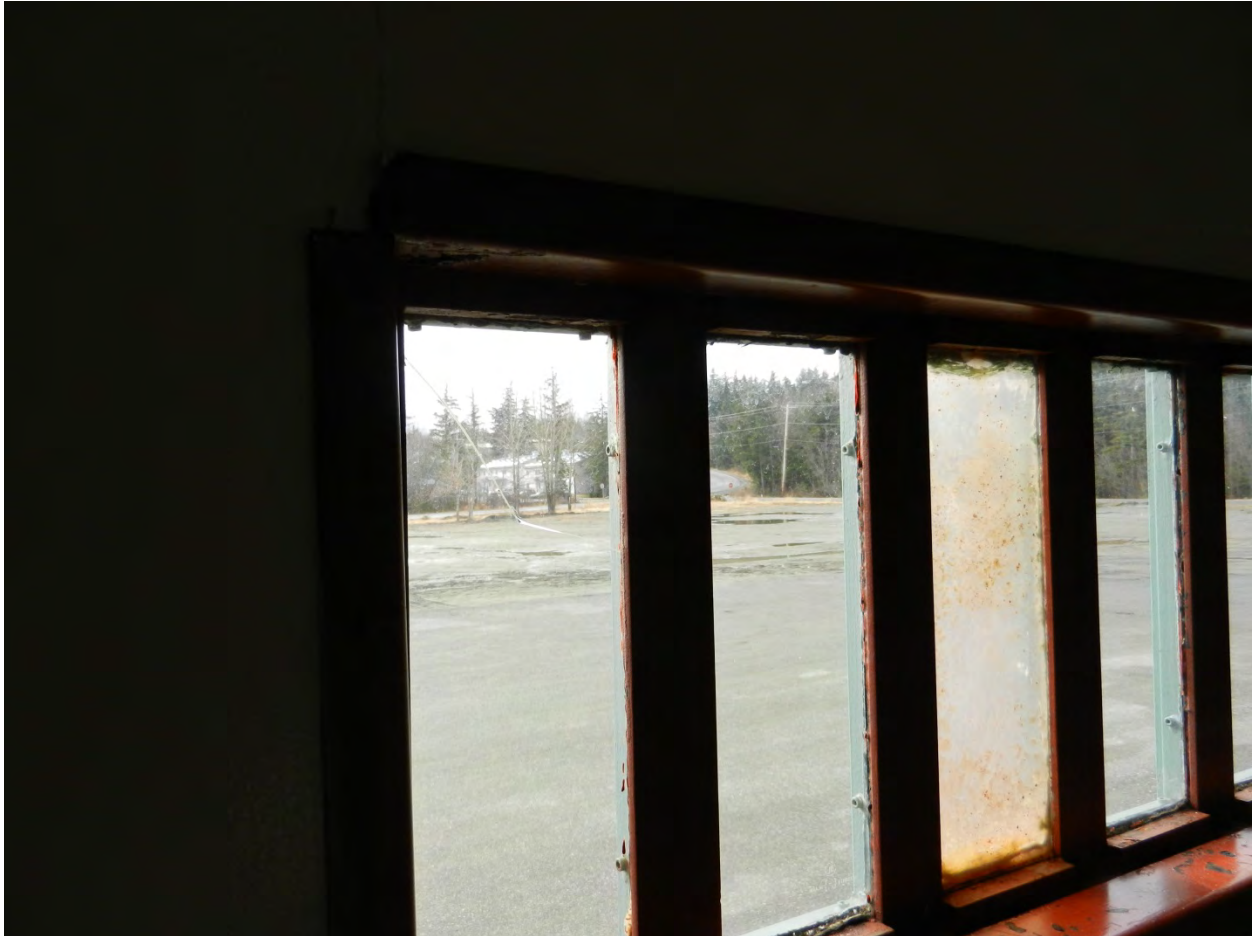
Photo 34 – interior of jail cell, cracked Plexiglass
