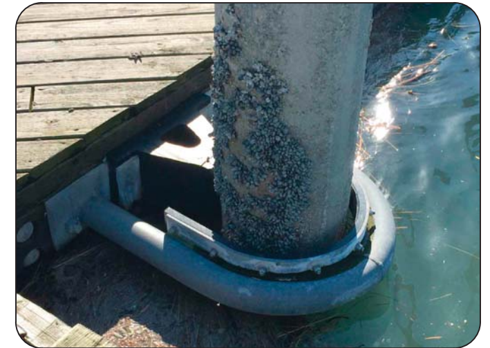
D SEAPLANE FLOAT PILE HOOPS TO BE REMOVED, SALVAGED AND REINSTALLED BY CONTRACTOR; FLOAT RELOCATED AND REINSTALLED BY OWNER
