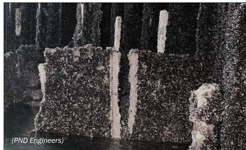
Figure 7: Corrosion Failure of the Interconnecting Closure Arc
