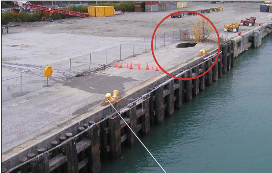
Figure 11: Sink Hole at Lutak Dock
