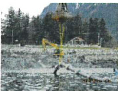
Heritage Harbor Outfall
