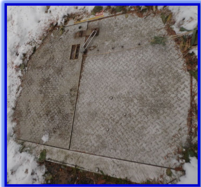
Figure 4.4: Beach Road Lift Station, 2022
