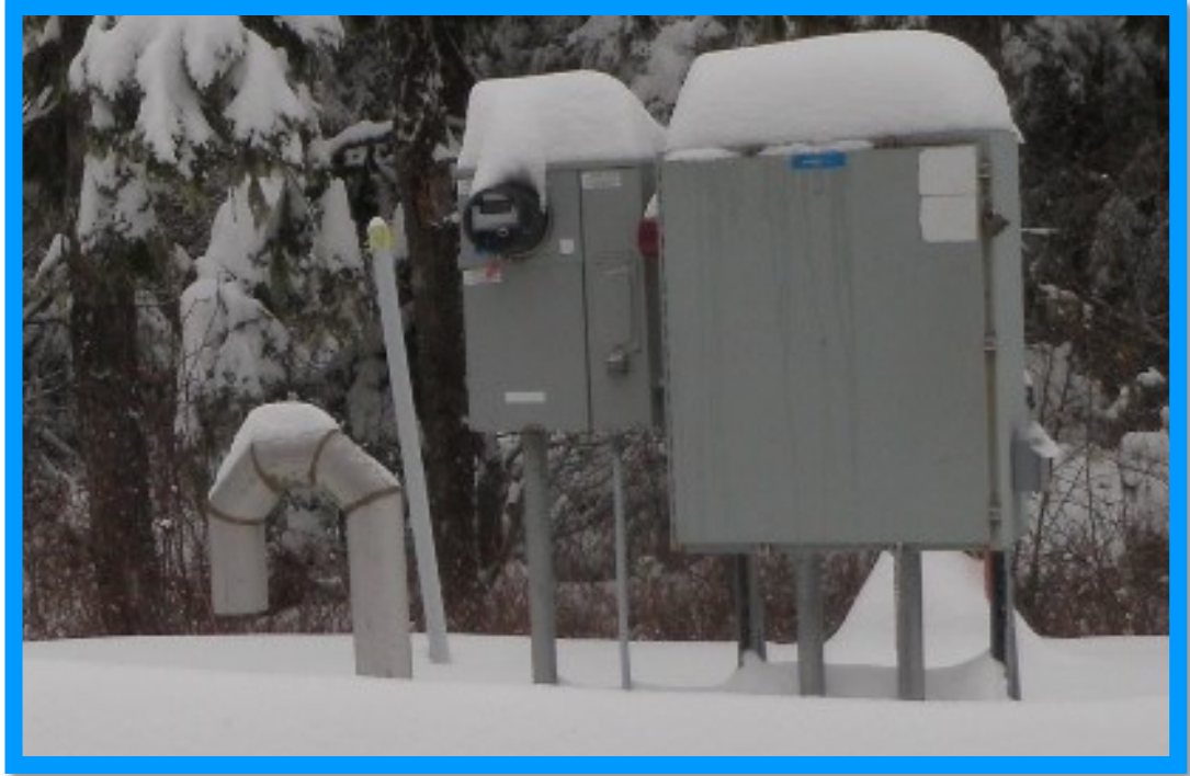
Photo 10 & 11: Chilkoot Estates Lift Station
