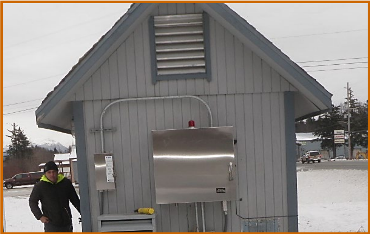
Figure 1.1: Controls for One-Mile Lift Station with Utility Supervisor
