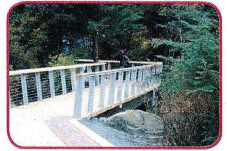
Identifying permitting issues at the onset allows the planning effort to be responsive. (Sitka Seawalk and elevated boardwalk over wetlands)
