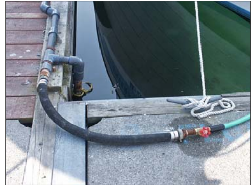
Harbor Water System
